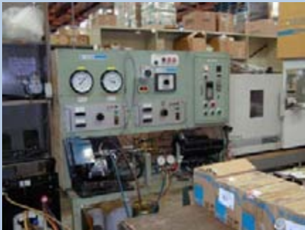
Sanden warranty testing equipment.
